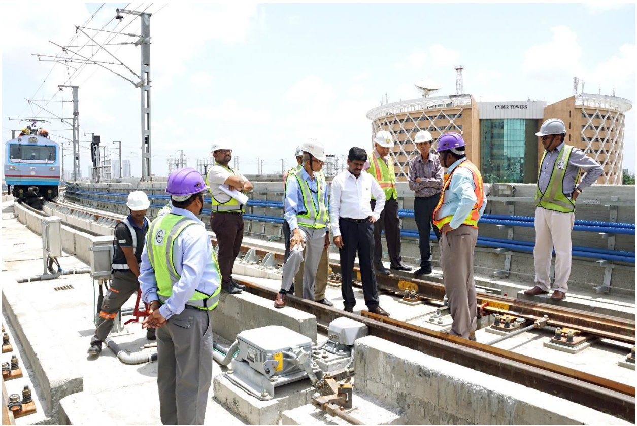
Image 1 - Mr. DVS Raju, CEIG along with other officials inspecting the track works
