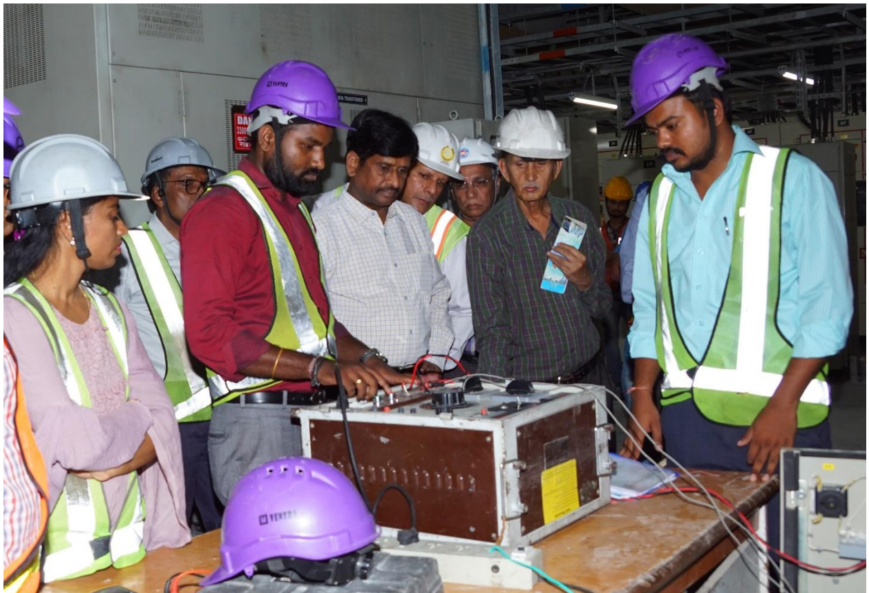
Mr. DVS Raju, CEIG along with other officials inspecting an auxiliary substation.
