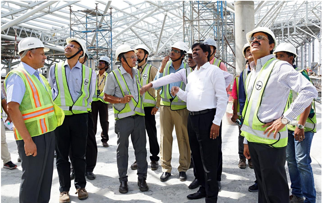
Mr. DVS Raju along with other officials inspecting the OETS at MGBS Interchange Station.
